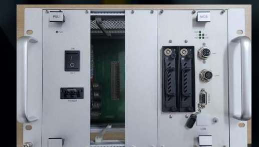
CCTV Broadcasting system (NVR) Phison S12DI SATA SSD Inside
